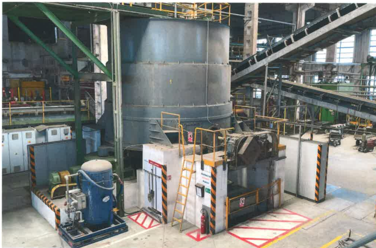
2 | Production mixture silo
